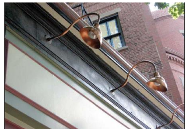
Gooseneck light fixtures are recommended to illuminate signage
